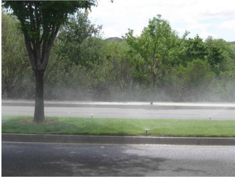
Station 25: Non LittleValve area Excessive misting and overspray
